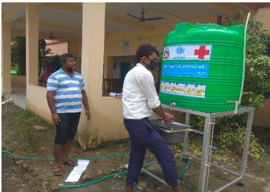
Figure :Contactless hand washing station installed in Shree Judda higher secondary School, Gaur-2, Rautahat
